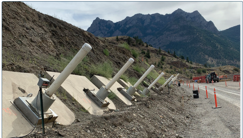
Load Cells installed on multi-strand ground anchors monitoring stability of landslide.
