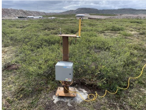
Figure 11: Example of GNSS Base Station Control Box Configuration Field Installation
