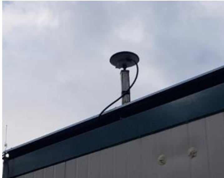
Figure 9: GNSS Antenna Example Installation
