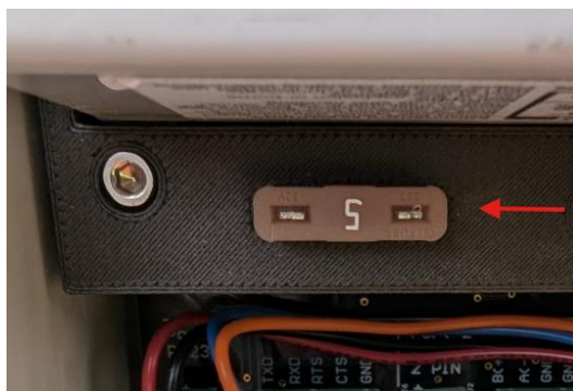
Figure 14: Fuse Inserted into Battery Module
