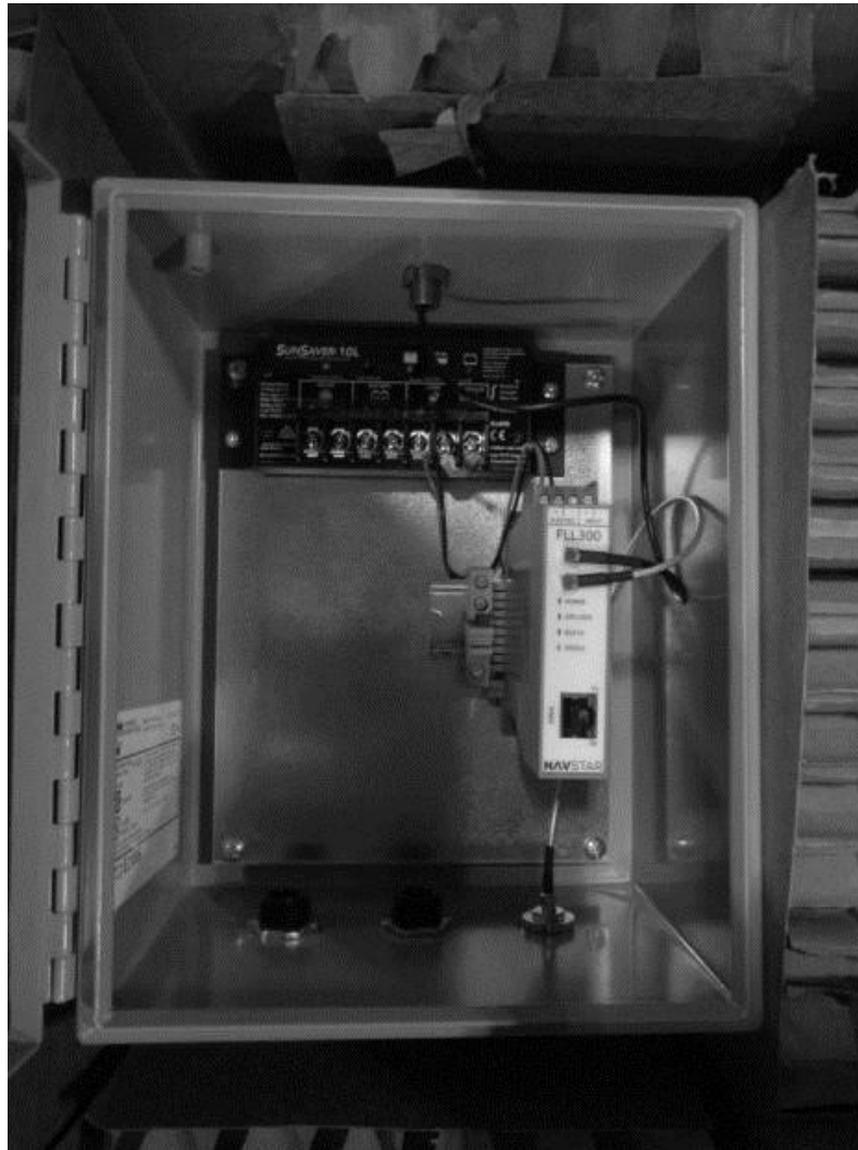
Figure 3: FLL300 Repeater box with solar controller
