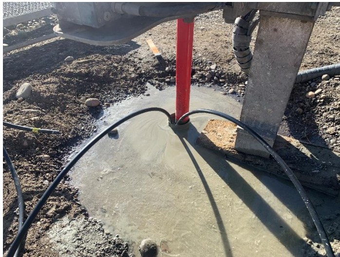
Figure 10: Pumping Grout through the Grout Pipe to Set the Casing Assembly in Place
