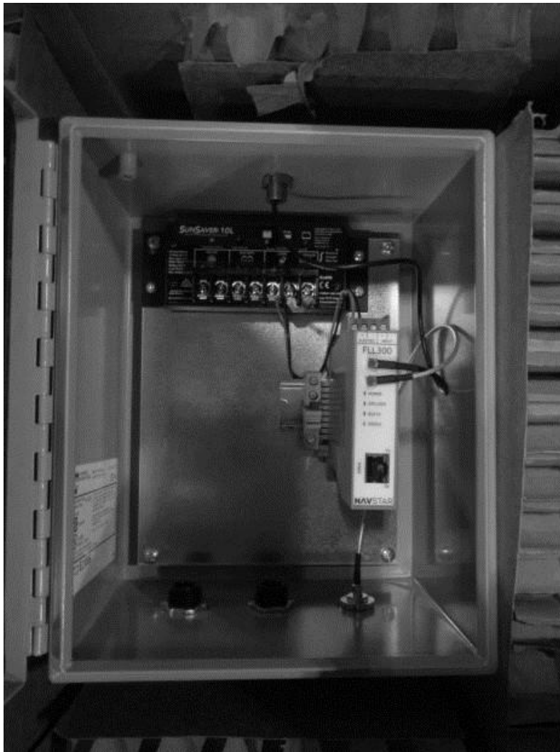
Figure 3: FLL300 Repeater Box with Solar Controller
